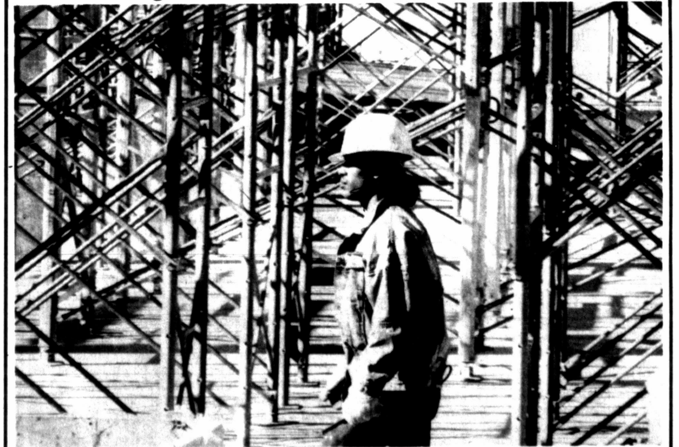
Ralf Felix, a worker on the construction of the new Gray County Jail and Sheriff's Office, walks by a maze of gridwork at the site Friday. The gridwork is shoring and bracing to support the formwork of the second floor. Estimated completion date of the new facility is late November.
