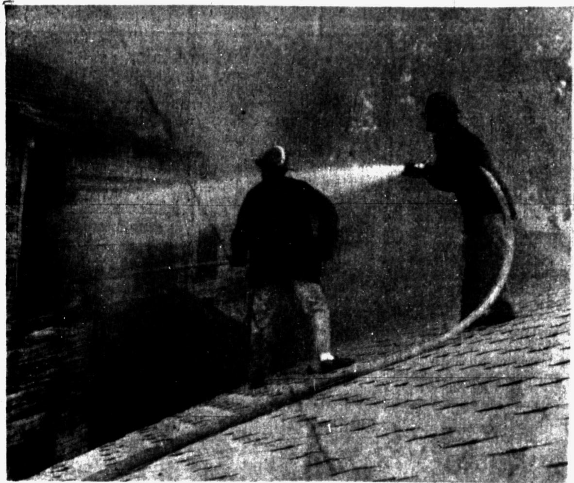
GUTTED IN FIRE —A fire which broke out at 3:11 p.m. Friday gutted the inside of the upper story of this two-story frame building at 405 Maple St. on the city's south side. The lower floor suffered heavy smoke and water damage. The upper floor contained a rooming house and the lower floor housed a barbecue eating place and a pool hall. Firemen fought the blaze for about two hours before bringing it under control. No injuries were reported and no estimates of damage were available.
