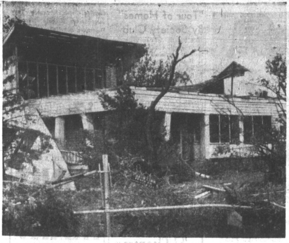
STORM DAMAGE — This house, across the street from the school building in Miami, suffered heavy damage in Monday's tornado which injured five persons. The house was thought to be unoccupied at the time of the storm and the damage is representative of that dealt to a number of homes in Miami.
