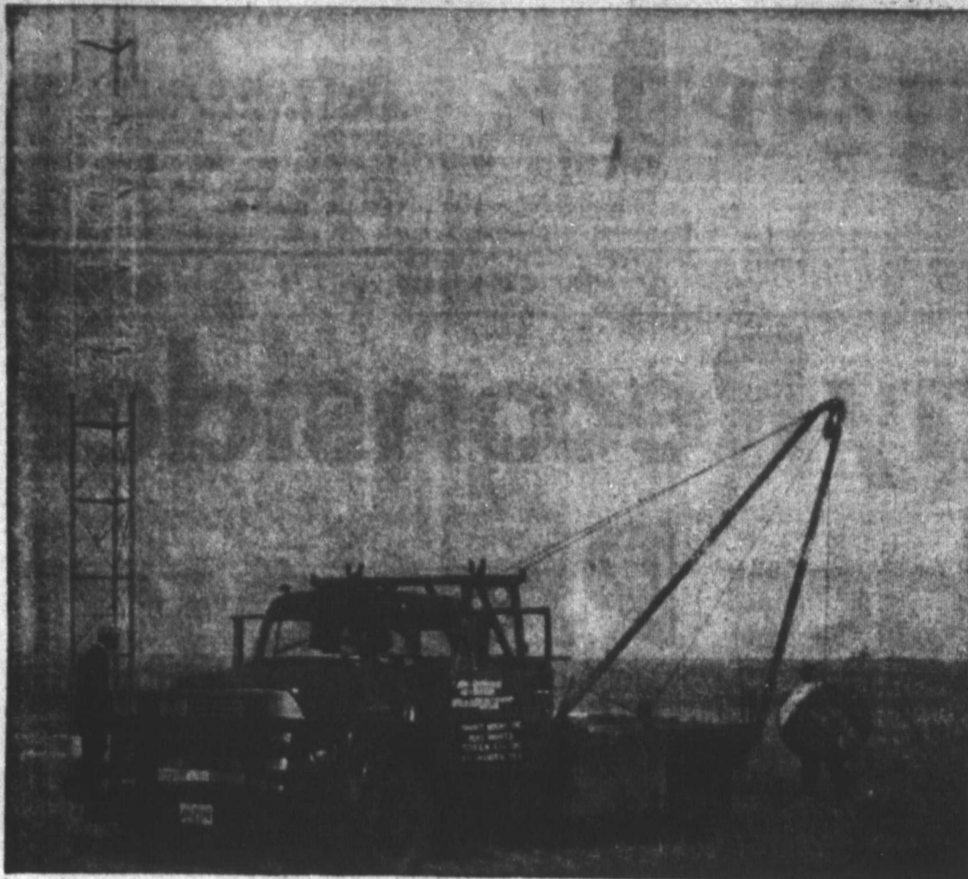
MORE CABLE TV — Workman for the Fort Worth Tower Co., are shown here yesterday as they installed the micro-wave tower that will add two new channels for Pampa Cable TV viewers. The 132-ft tower will bring in programs from Channel 39 in Dallas and Channel 11 in Fort Worth and will be in service by Oct. 1. They will be received in Pampa on Channels 2 and 5, according to Wayne Stedum, local Cable TV manager.
