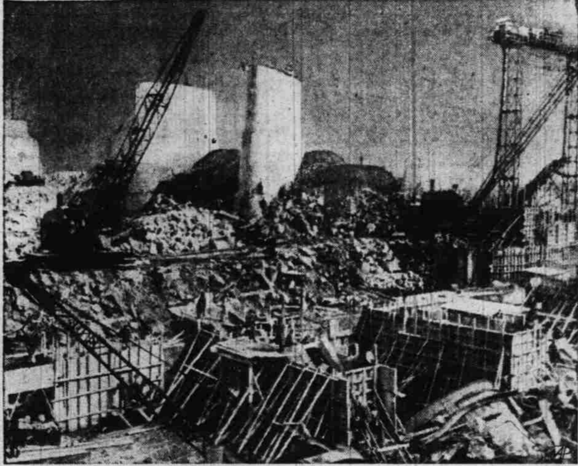
RUSSIANS REBUILD DAM—Forms are ready to receive cement as Russians rebuild a large Dnepr river dam, near Dnepreptovsk, destroyed by the retreating Red army in 1941.
