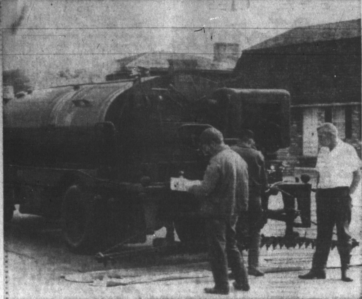
SEAL COATING PROJECT PROGRESSES—A crew of Lewis Construction Co. workers, left to right, Bob Barker, Allen Barker, and Bill Noel, all of Dumas, moved with the seal-coating equipment today to streets north of 23rd, including Aspen, Christine, Mary Ellen and Charles as the annual seal-coating project progressed. (Staff Photo)
