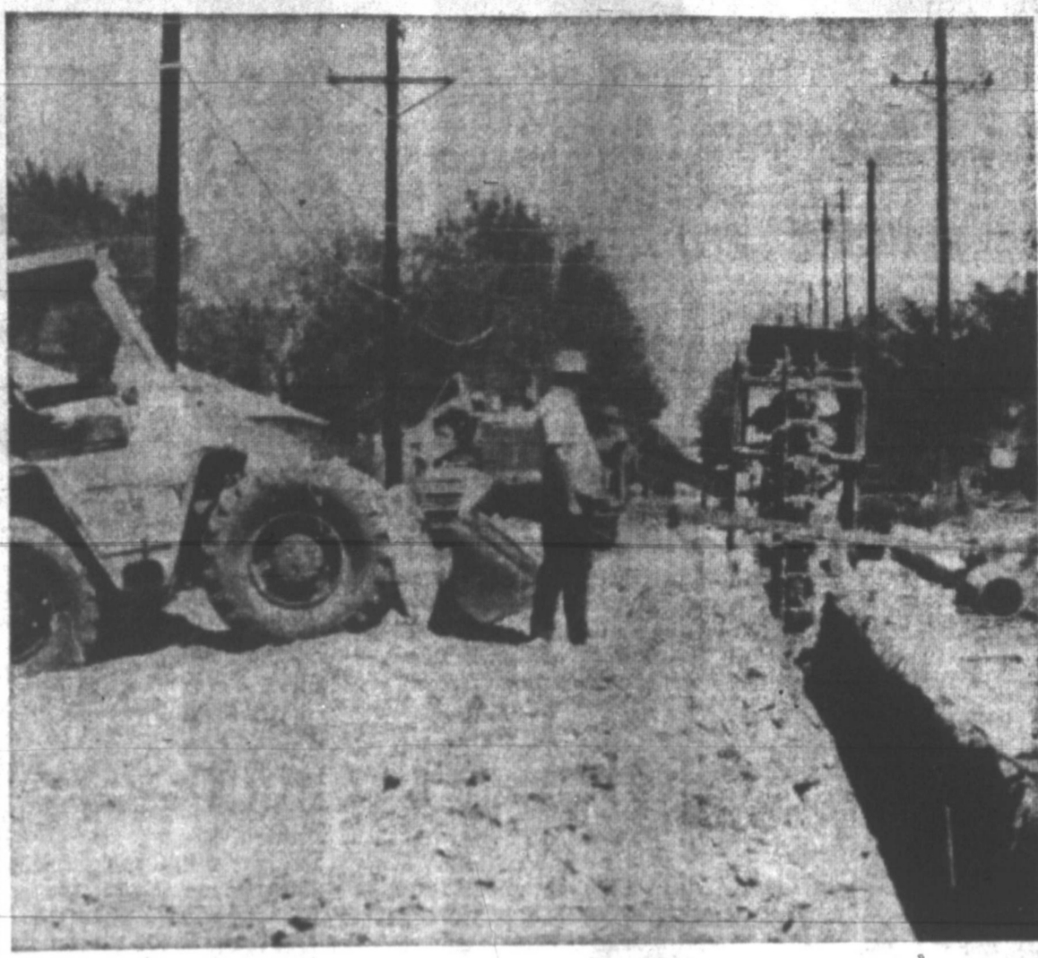
CONSTRUCTION continues for Pampa's new water distribution system with installation of a pipeline from the new water treatment plant on W. Kentucky, eastward to Lefors St. Projected completion date for the work is August with the actual influx of treated Lake Meredith water expected early next year, according to Wayland Merriman, engineer. Construction is under supervision of Merriman and Barber Consulting Engineers Inc. (Staff Photo.)
