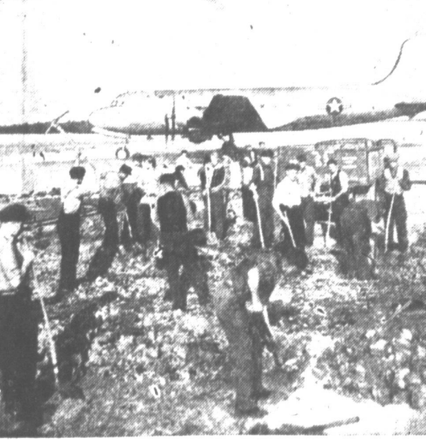
Gatow Airfield, in the British sector of Berlin, is being expanded to handle more aircraft. Already, some 400 planes fly about 3000 tons of supplies over the Russian blockade daily. German laborers lay foundation for a new strip, while a C-47 lands in background. (Photo by NEA-Acme staff correspondent Erich Engel.)
