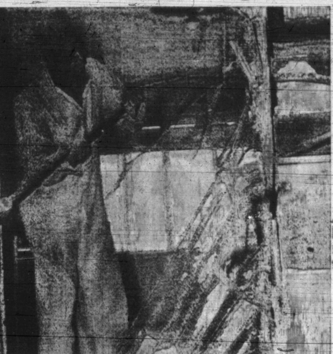
TEARING IT DOWN — Tom Morgan, Pampa, part of a construction crew that started work this morning on the District Court Room, begins work with his sledge hammer, tearing down walls on the court balcony. Air conditioning, a new jury room, a new client-lawyer room and new tile and lowering of the ceiling is planned for the courtroom. (See Story, Page 1).
