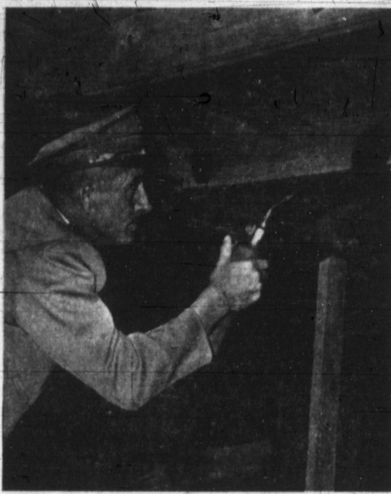
FIREBUG? — Pampa Fire Marshal L. V. Bruce attempts to start a fire in the attic of the Casa Del Nursing Home but to no avail. The attic had just been sprayed with a chemical solution making it fireproof.
