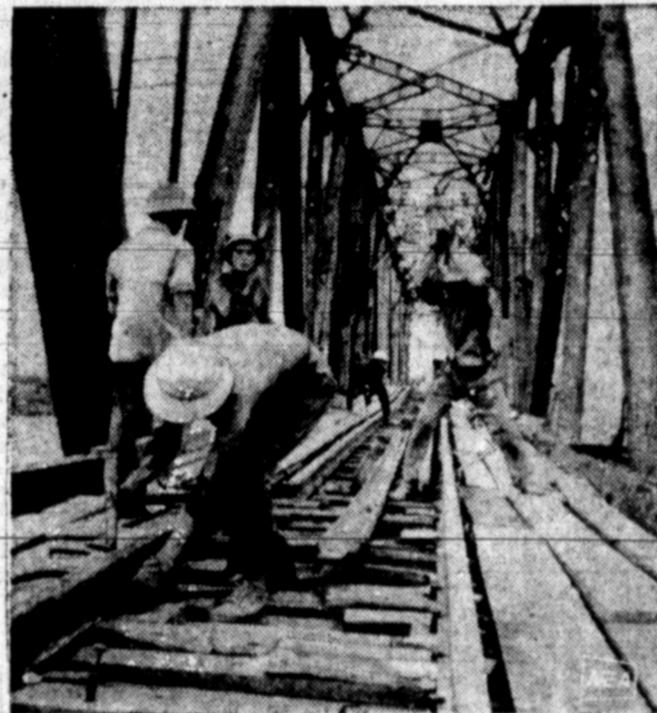
BRIDGE REPAIR in North Vietnam goes on continually to keep supplies flowing to Viet Cong and North Vietnamese in South Vietnam, according to this photo and caption material from a Japanese news service. This unidentified bridge has been attacked and damaged numerous times by American planes, but never completely destroyed, the North Vietnamese claimed.
