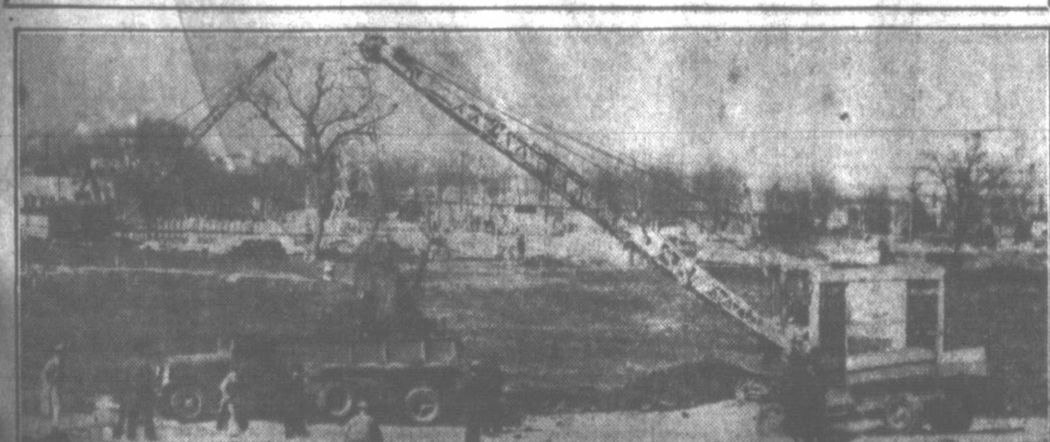
Workmen are laboring in three shifts on excavation of the huge cultural center at the Texas Centennial Exposition. The start of the excavation, opposite the site of the Ford Exhibit Building, is pictured in the photograph above.
