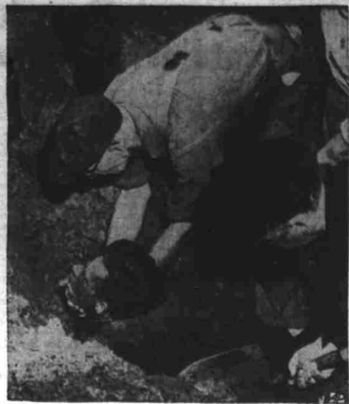
Trapped In Cave-In Rescuers dig soft mud from around Stanley W. Pakel Jr. of Johnson City, Tenn., after he was trapped and completely covered by a cave-in in the ditch in which he was preparing to lay a sewer pipe at Binghamton, N.Y. Fellow workers dug mud from around his head with their hands to keep him from suffocating. (AP Wirephoto).
