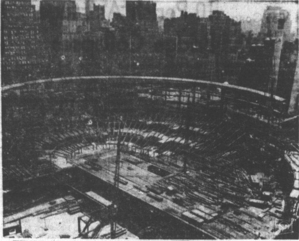
THE NEW MADISON SQUARE GARDEN is beginning to take shape among the buildings of midtown Manhattan. The steel skeleton of the huge new sports arena is going up where Pennsylvania Station once stood.
