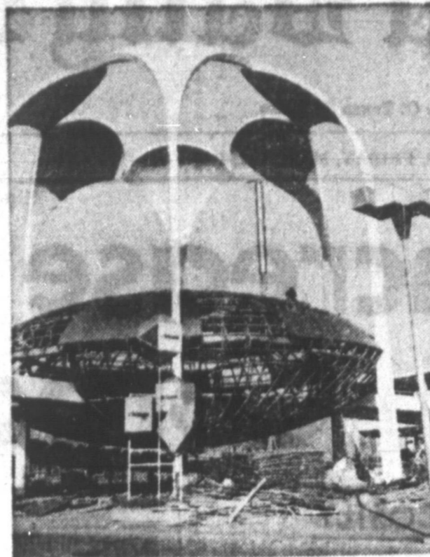
While traces of the World's Fair rapidly succumb to the demolition worker at Long Island's Flushing Meadows, not all of the fanciful pavilions and halls which intrigued visitors during the fair's two-year run are destined for the scrap
