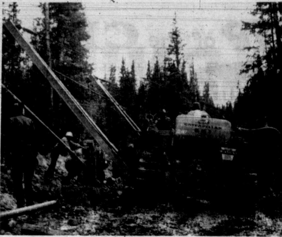
GOING UP AND UP — Workmen from McCathern, Inc. of Pampa are digging ditches and putting in a gas pipeline in Summit County, Colorado. The men finished putting in the world's highest gas pipeline in October.
