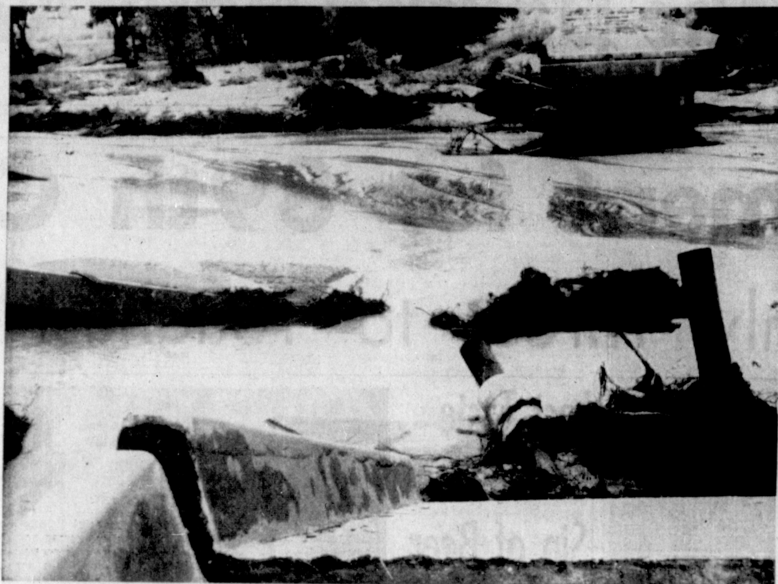
WATERSHED NEEDED — Flood waters rampaging down the McClellan destroyed this newly constructed bridge several years ago. This is just one of the reasons farmers and ranchers in Gray and Carson counties rolled up their sleeves and went to work to secure a $1 million
