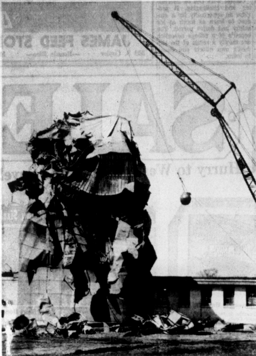
BUILT TO LAST —The wrecker's ball took its toll of this old silo, but not before the old structure put up a good fight. Progress won another battle.
