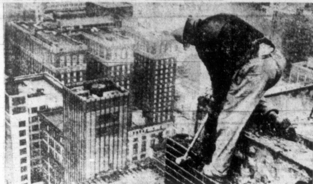
BEGINS DEMOLITION — More than 520 feet above street level, a workman begins a brick-by-brick demolition job on the roof of the Morrison Hotel in the Chicago-Loop. The world's tallest hotel, the Morrison is being razed to make room for a new 60-story building which will house the First National Bank.
