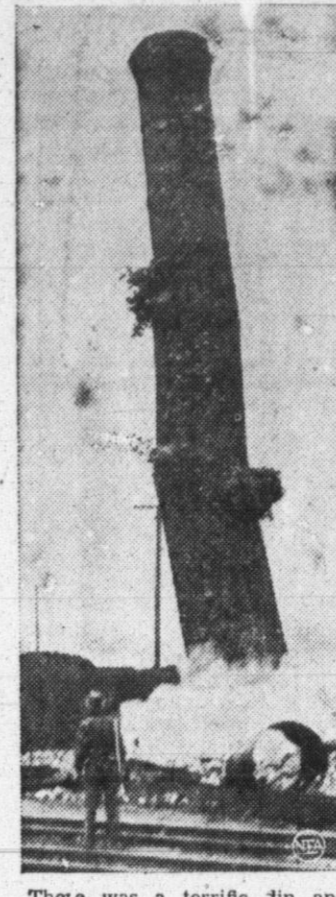
There was a terrific din and bricks spewed in every direction a few seconds after this picture was taken of a chimney literally tumbling to destruction in Peoria, Ill. Workmen chiseled out a few bricks at the base, the tall figure swayed, bent, crumpled, crashed.
