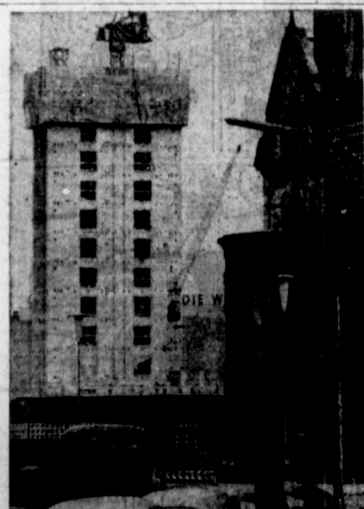
WEST BERLIN ABUILDING —Work is rapidly progressing on West Berlin's newest building project, the 22-story Europa Center, a huge complex of offices, apartments and shops in the heart of the city. It will be the tallest building in West Berlin. To the right is the Memorial Church.
