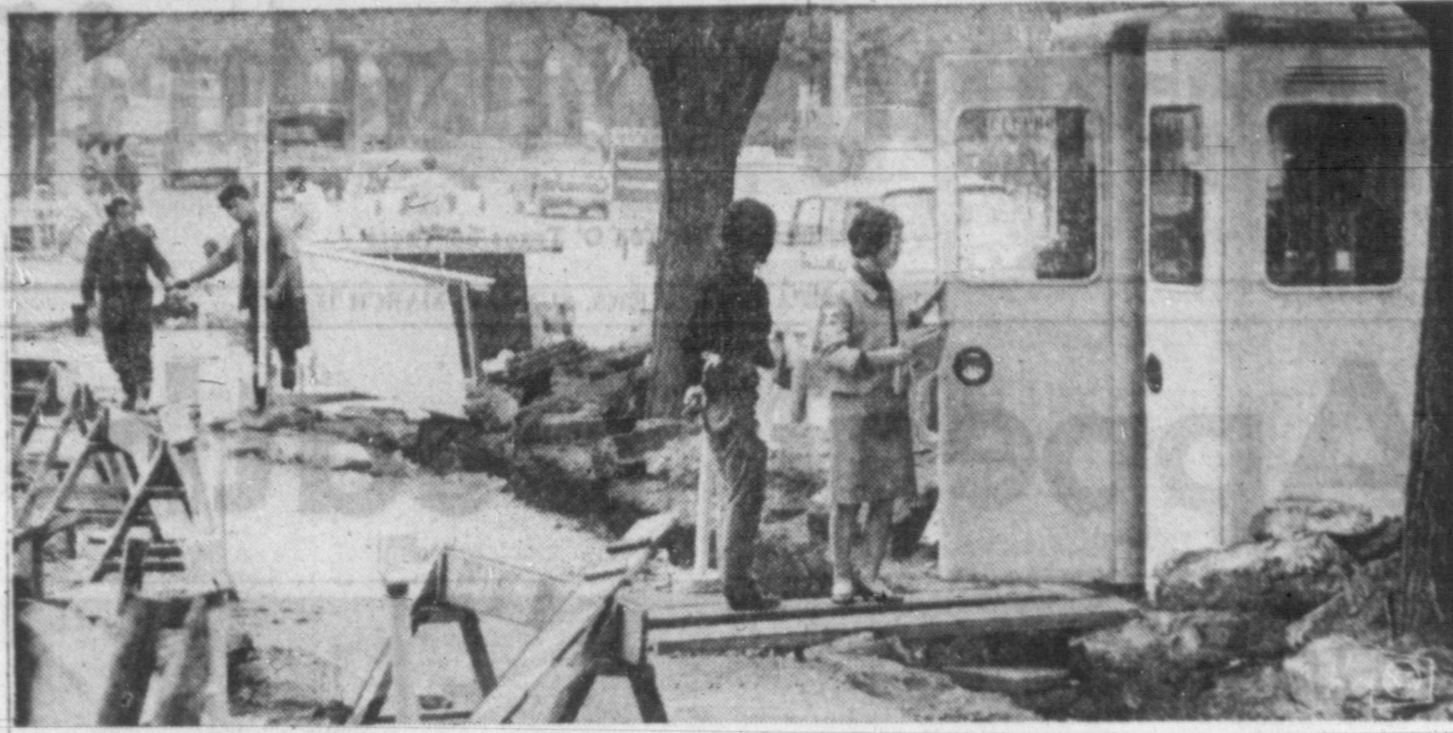
ALL THIS FOR THE OLYMPICS —To put their city in shape for the 1964 Olympic games in October, residents of Tokyo are ripping it apart. And, in a city of more than 10 million people, this flurry of repairing and construction is causing some problems. Traffic congestion in normal times is a problem, but when streets and sidewalks are torn up, residents are confused. To accommodate Olympic throngs, the Japanese are building a subway and more highways. In the above photos, even making a telephone call is hard. These girls have to walk a plank to reach a booth.
