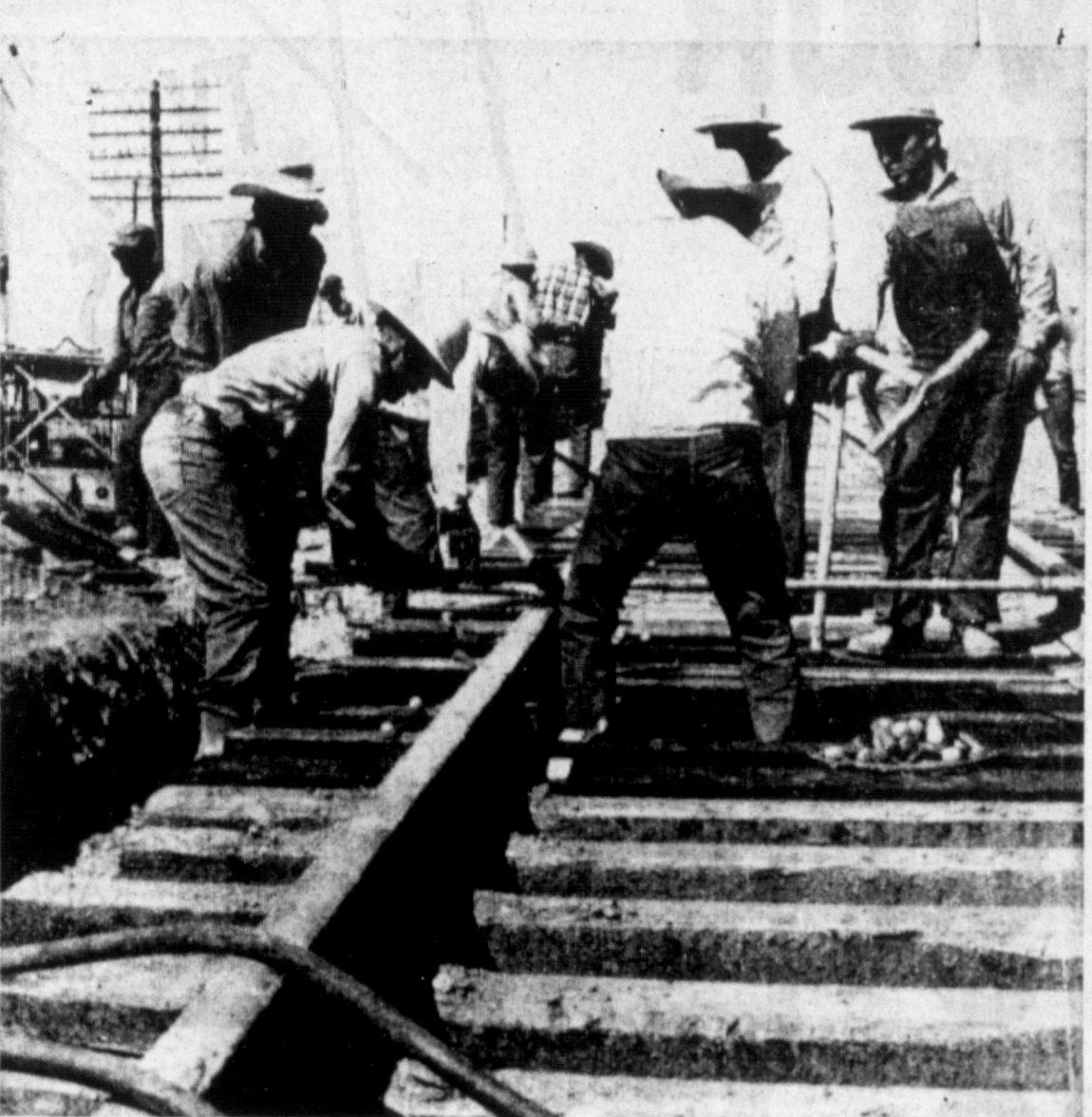
ROAD CLOSED — Price Road, west of Pampa, was closed to through traffic today while Santa Fe Railroad track crews rebuilt the two-line crossing. Railroad officials said the double tracks from Pampa to west of White Deer will be rebuilt during the next few days. New ballast is being added above and new ties put in place. The north end of Price Road remained open to allow access to business establishments. (Daily News Staff Photo)
