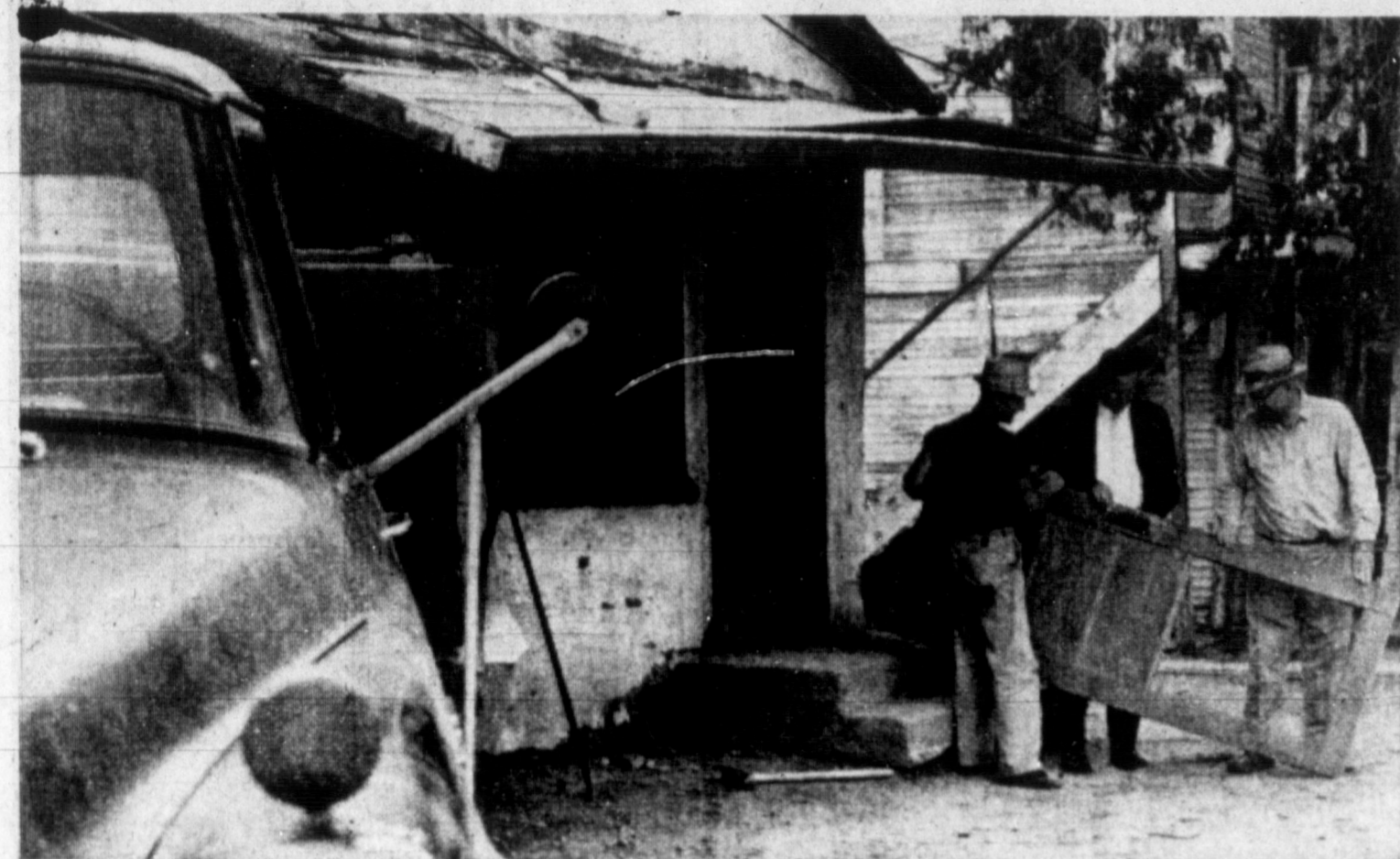
FIRST OF 25 — Work of dismantling one of 25 dilapidated, tumbledown buildings in Pampa was started yesterday at 401 Maple. Shown here, left to right, are Jim Fleming, street department employee; Warren Fathree, chairman of a Chamber of Commerce committee working
