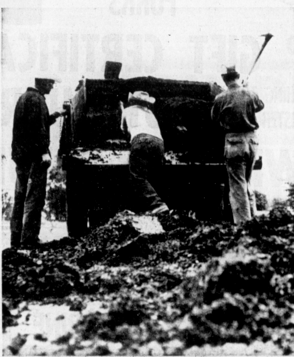
PATCHING — Texas Highway Department employees have begun a patching and leveling project on Hobart St. in preparation for the new surface scheduled to be added this summer. Low places in the paving and rough spots are receiving the treatment shown above. Cold-mix surfacing is dumped on the street and rolled, to improve the street and make it more suitable for the hot-mix asphalt which will be added later.
