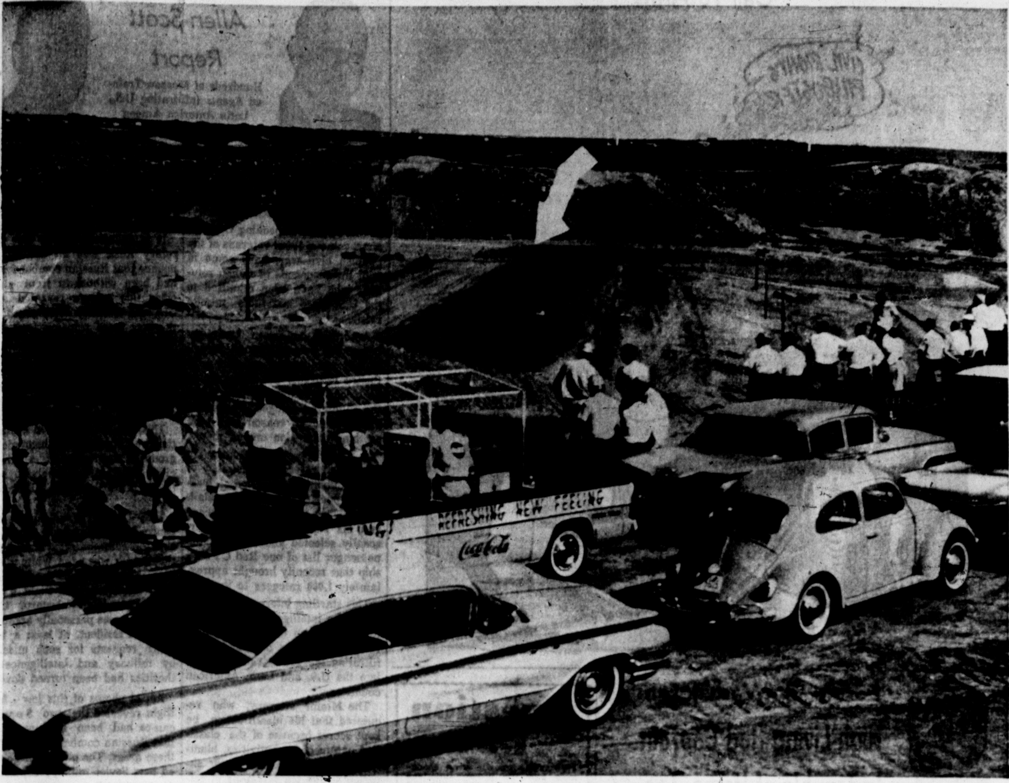
PAMPA TOURISTS INVESTIGATE DAM PROGRESS — Pampan who participated in the Chamber of Commerce tour of the Canadian River Dam site at Sanford yesterday are shown looking at the excavation for the base of the dam, left arrow, and the water diversion
