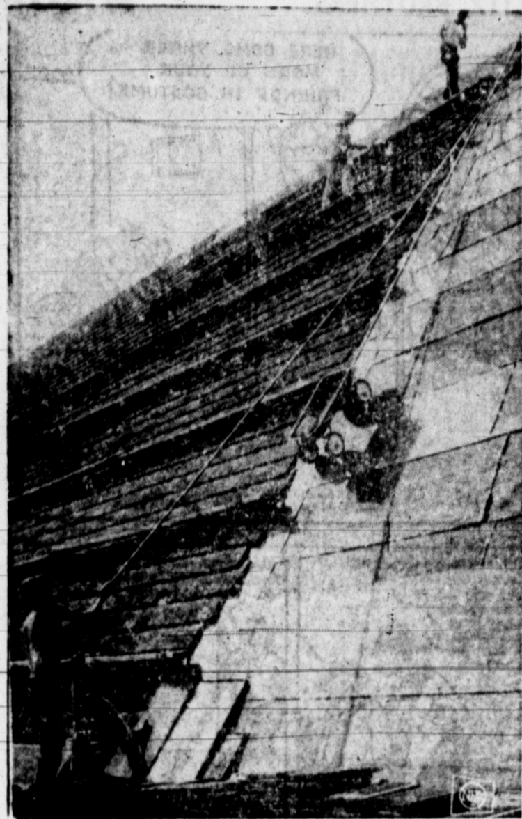
WAGON'S NEW USE —The little red wagon has long been a child's favorite, but these Topeka, Kan., workmen have found a new use for it. They use it as a lift, helping to raise supplies to those perched high on a steep church roof.
