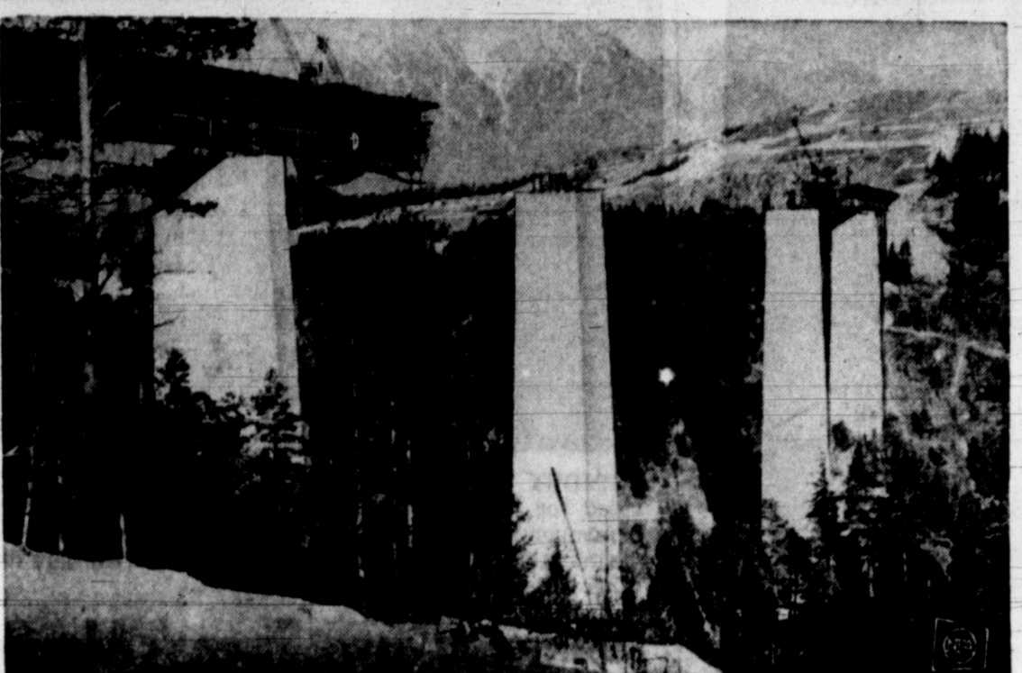
UP IN THE VALLEY—The Europa Bridge, destined to be the biggest bridge in Europe, inches its way across the Wipp Valley near Innsbruck, Austria. To be completed in time for the 1964 Winter Olympic games at Innsbruck, the 2,000-foot-long bridge will carry five lanes of traffic 600 feet above the valley floor. In background are peaks of the Nordketten Range.
