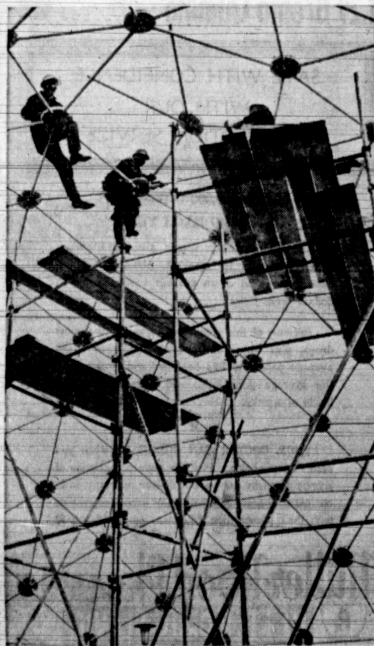
WEB-TIED —Seemingly caught in a giant spiderweb, workmen scramble atop a constructed pattern of steel to connect the shell of a modern tent pavilion at West Berlin. The structure appeared at the German Industrial Exhibition.
