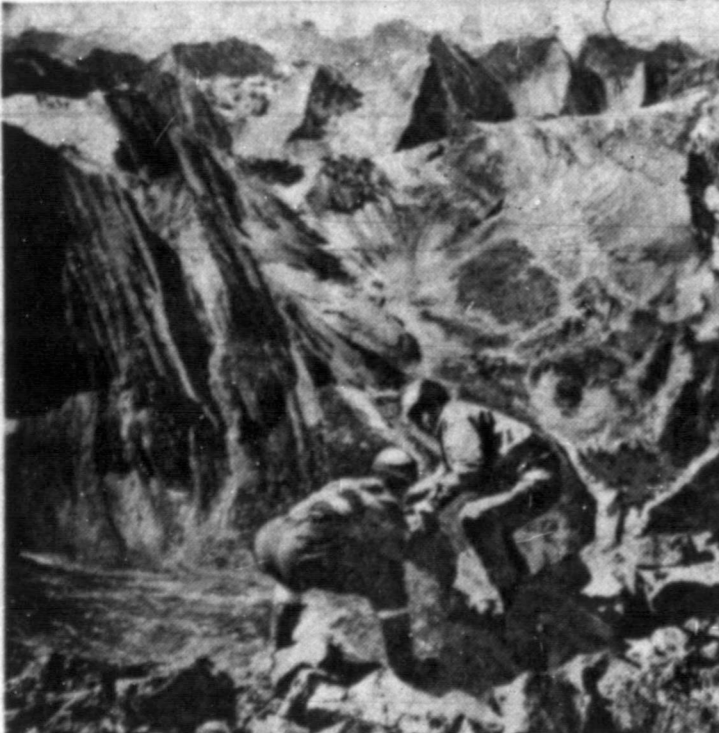
LOOK OUT BELOW! —Rock disposal is no problem at the microwave relay site atop Pyramid Mountain in Canada's Jasper National Park. Workers merely roll boulders over the edge. Some 30 feet of the summit is being sheared away for a communications tower.
