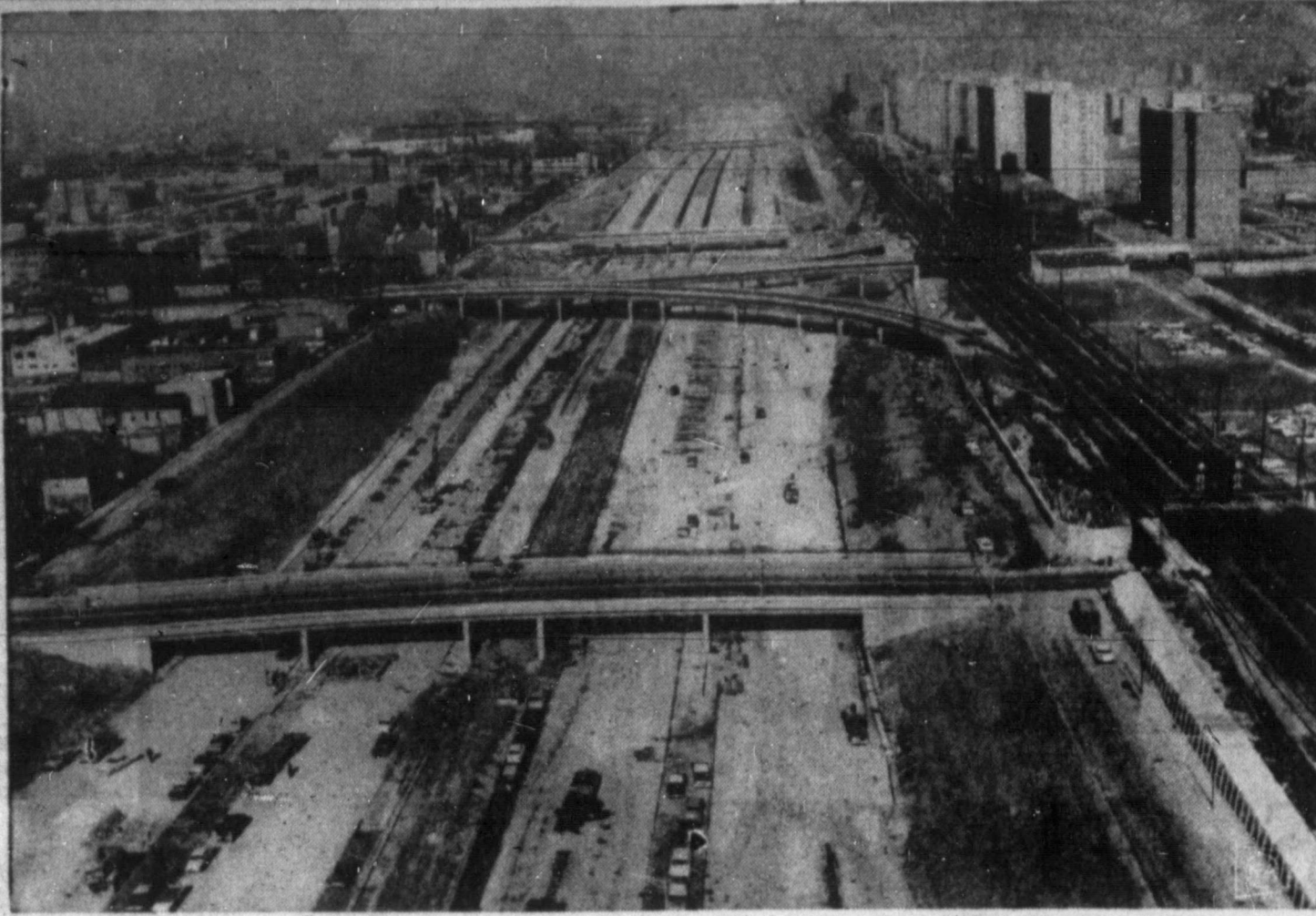
WORLD'S WIDEST—Aerial view shows progress of construction on the world's widest superhighway, the Dan Ryan expressway, which runs 20.8 miles through Chicago's south side. The expressway will carry 16 lanes of traffic.
