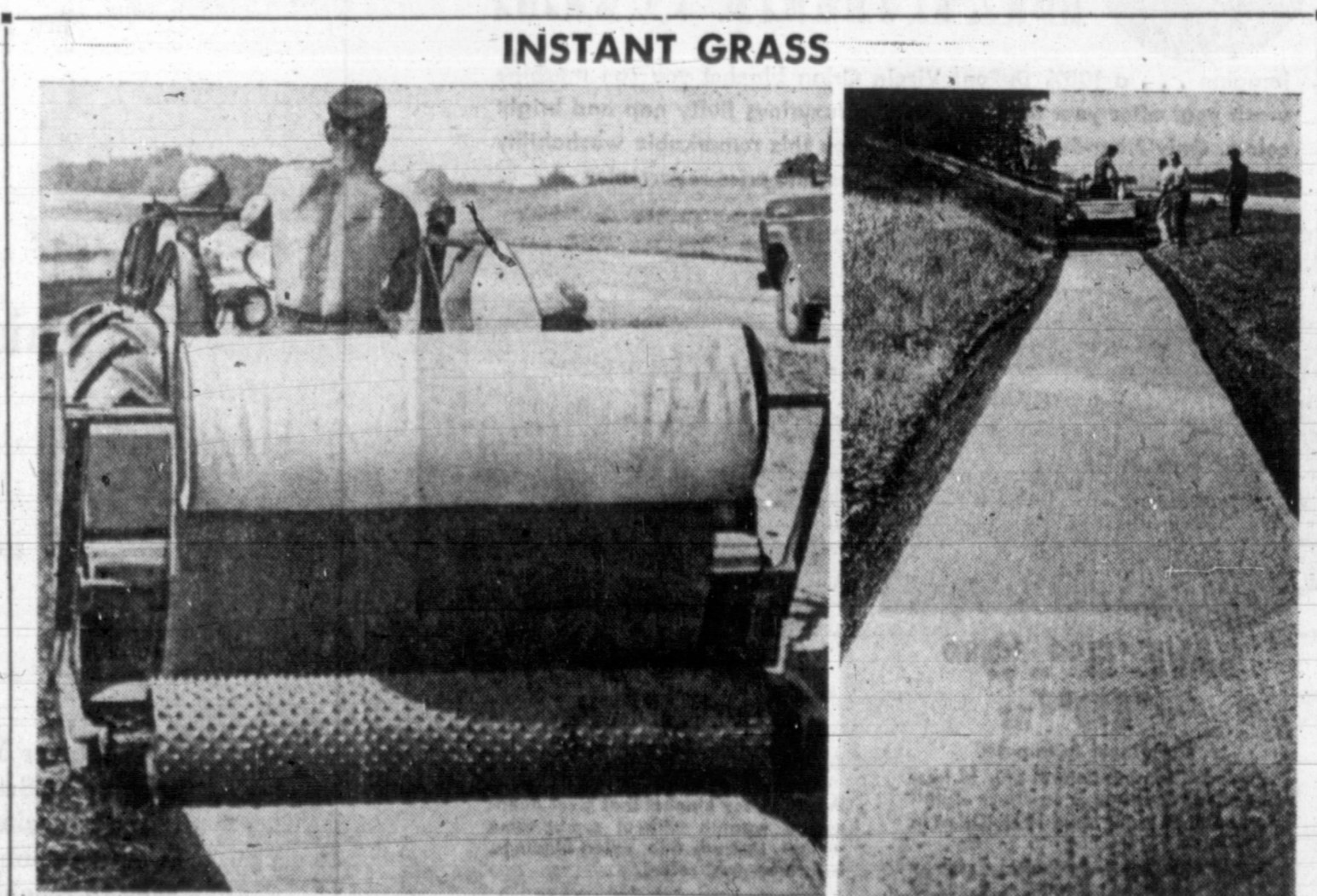
GRASS ROOTS CAMPAIGN —Unrolled like paper toweling, a new "instant grass" carpet was installed along U. S. Highway 90, near Mentor, Ohio. The 1,000-foot-long, 4½-foot-wide carpet, a mat impregnated with grass seed and fertilizer, took just two weeks to produce grass at half the cost and time of conventional methods. The mat construction allowed the "gardener" to install the carpet on slopes of up to 85 degrees without danger of washout or erosion.
