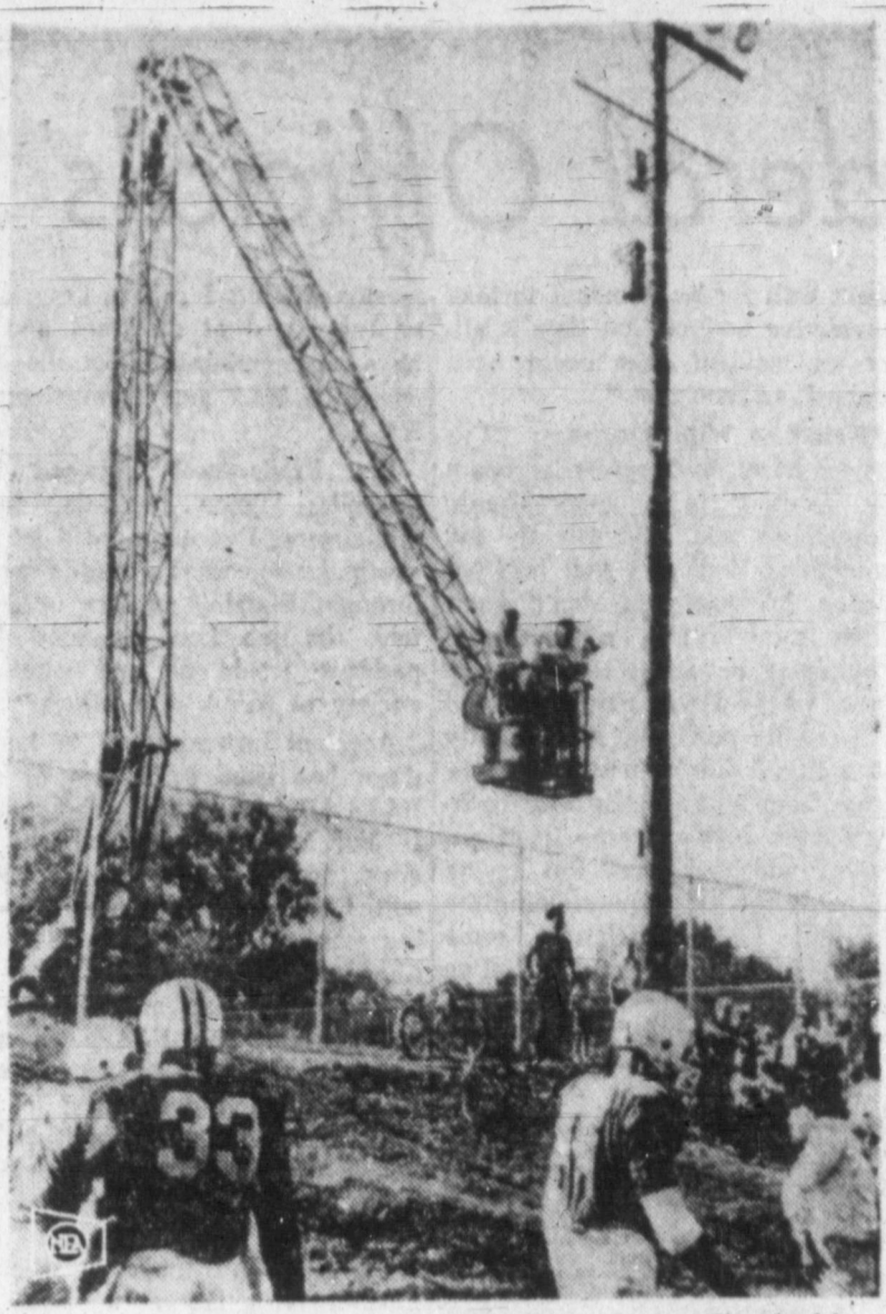
HIGHER EDUCATION—Coach Bob Blackman directs his Dartmouth football squad from the cockpit of an extension ladder truck, used for construction of a new fieldhouse.
