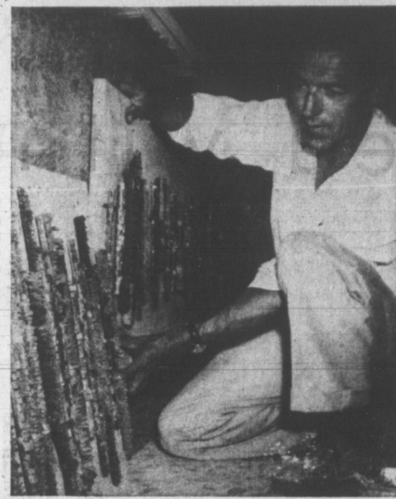
MOSAIC ARTIST AT WORK — Merritt Yearsley, one of the Southwest's most noted mosaic artists, is shown here while installing the modernistic design that underlines the tellers and cashiers' cubicles in the new Citizens Bank & Trust Co. lobby. The mosaic of copper and glass pieces on marble add greatly to the decor of the bank's interior setting.
