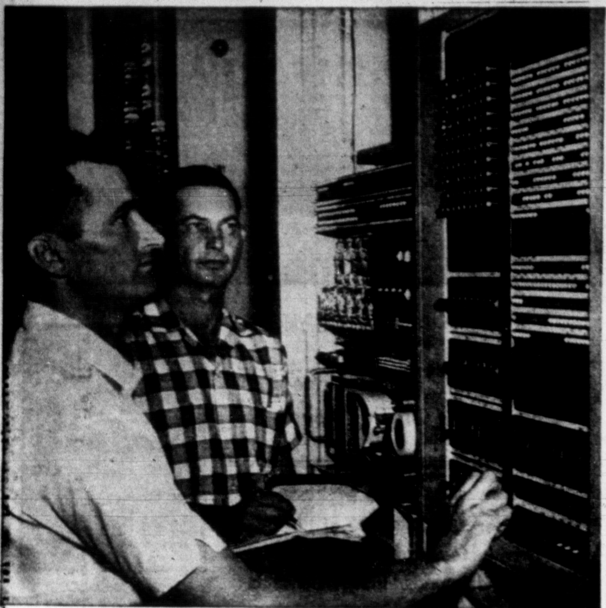
TELEPHONE PROGRESS — J. F. Allen, left, and A. W. Holt, Pampa switchmen for Southwestern Bell Telephone Company, operate the Pampa equipment for Bell's new direct distance dialing service. This machine, the automatic number identification frame, is used to locate and repair faulty connection and other trouble indications on the customer's line when he makes a DDD call.
