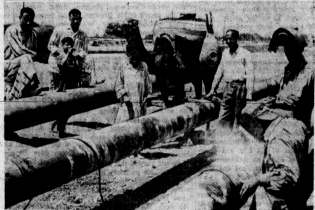
PIPELINE NETWORK —West German trained Egyptian welders, with a local audience, work on one of the three lines that will supply heating oil and kerosene to Egypt (bottom). Sitting on a kerosene pipe, one sidewalk superintendent (right) watches as the irreplaceable camels carry food and water to the workers (left). Phoenix Rheinrohr and two other German firms are building the network to open up the Nile Delta and pave the way for the growing Egyptian industrialization program.
