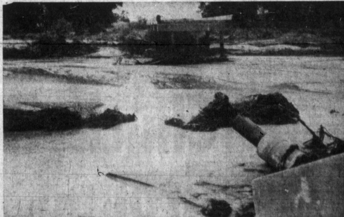
COULD THIS BE PREVENTED? — Shown here is the result of a flash flood on June 4, 1961, when this bridge was washed out on Highway 291 between Lefors and Alanreed on the McClellan Creek. A McClellan Creek watershed hearing is set for 2 p.m. Saturday in McLean to determine if the correct watershed structures could prevent such wash-outs as this. (Daily News Photo)
