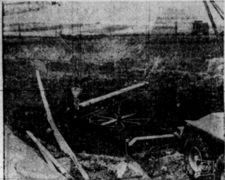
SILCO SENTINEL —Workmen gently ease the lower launching tube of a Minuteman missile into place in a huge hole in the rock beneath Montana farmland. Measuring more than 50 feet in length and 12 feet across, the tube weighs as much as seven large automobiles. Above this will be placed a doughnut-shaped equipment room and upper launching tube. The site will then be covered over. Over 100 such launchers are being installed in northern Montana.
