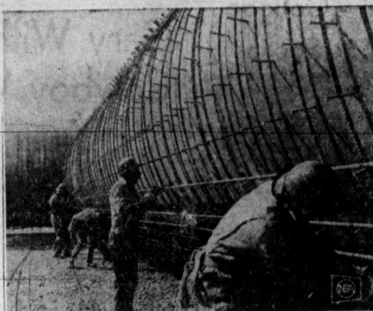
MINUTEMAN CAN —Huge lower launching tube liners, or "cans," are dressed up with two layers of steel reinforcing rods at American Bridge in Milwaukee before shipment to Minuteman missile sites around Malstrom AFB near Great Falls, Mont. Scores of the solid-fueled, nuclear bomb carrying intercontinental ballistic missiles will be stored underground to give the U.S. its first "hard" rocket striking force.
