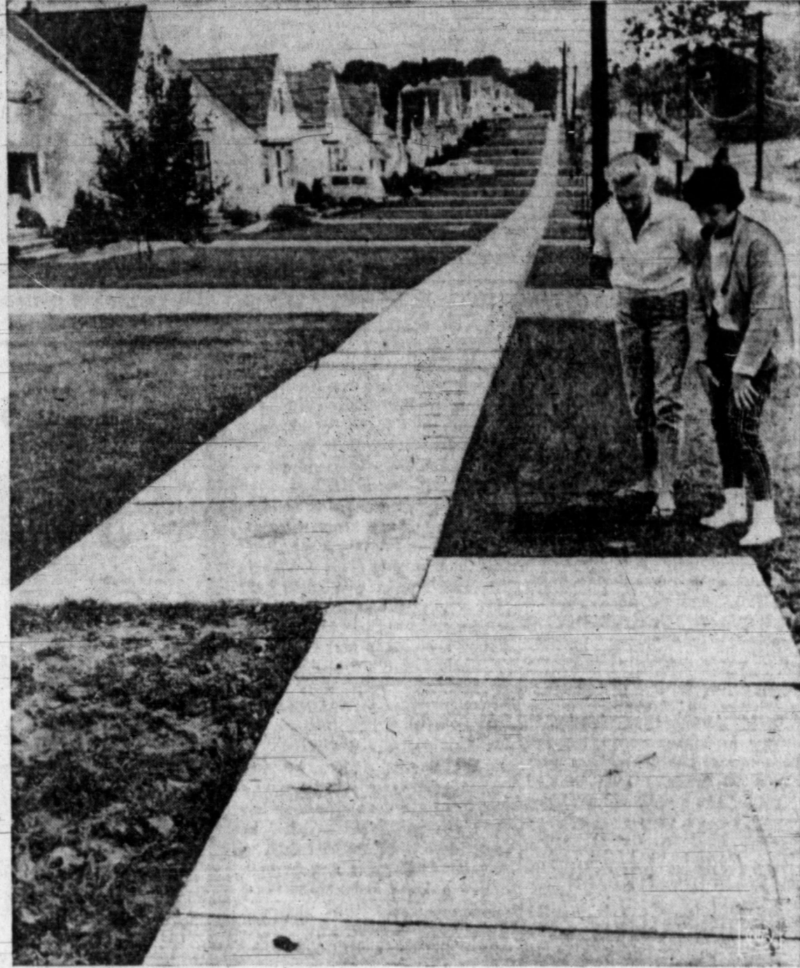
SOMETHING'S NOT QUITE RIGHT — Two Cleveland, Ohio, residents inspect the handiwork of two contractors — succumbing perhaps, to the feeling that somebody goofed.
