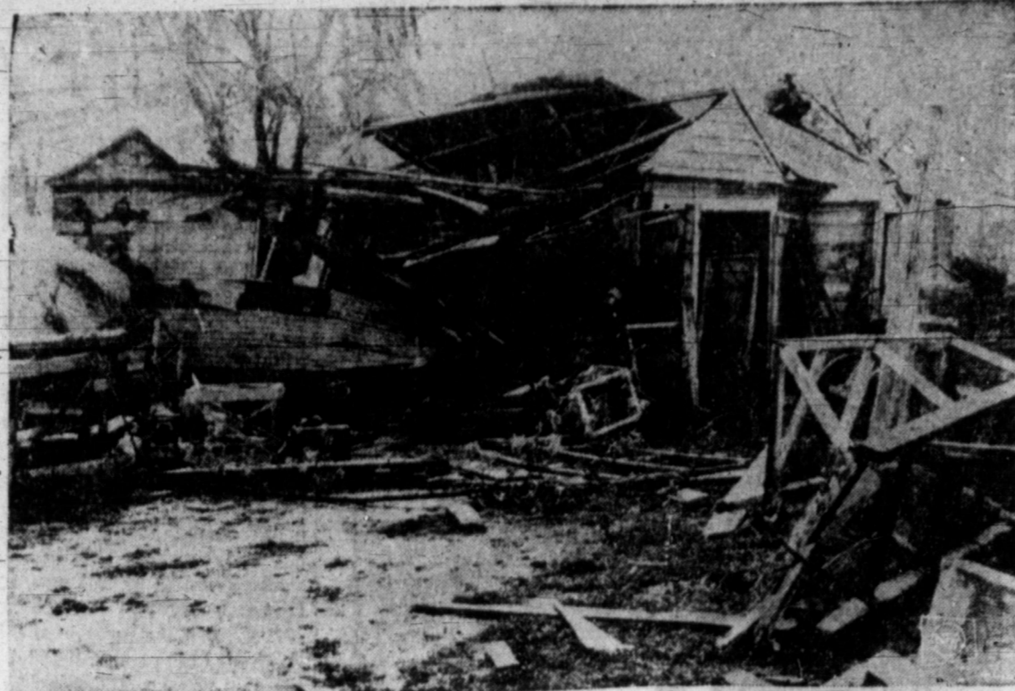
WEATHER DAMAGE — This was all that remained of the east end of the Thane Earle home near Whitewater, Wis., as a tornado, high winds and violent thunderstorms hit the Michigan-Wisconsin area.
