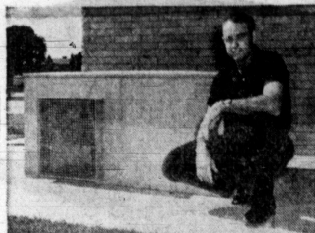
Mr. Smith poses next to 5-ton electric heat pump which adequately cools or heats the Smith's home—often times does both—during spring or fall when days are hot and nights are cool.
