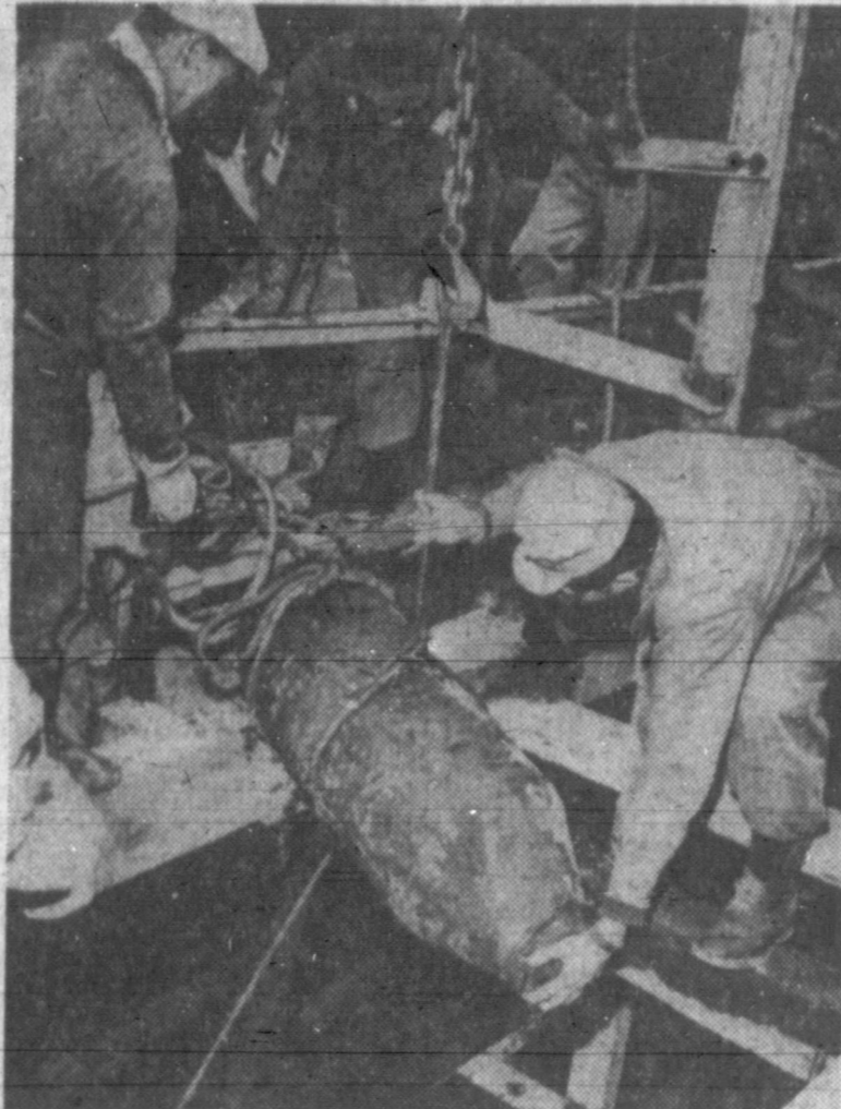
REMNANT FROM THE PAST —A wartime remnant is lifted by workmen from an excavation in Tokyo, Japan. The bomb was found 11 feet underground in a building site at Shinjuku Ward. The left-over was removed and defused by the Tokyo Self Defense Force bomb disposal unit.
