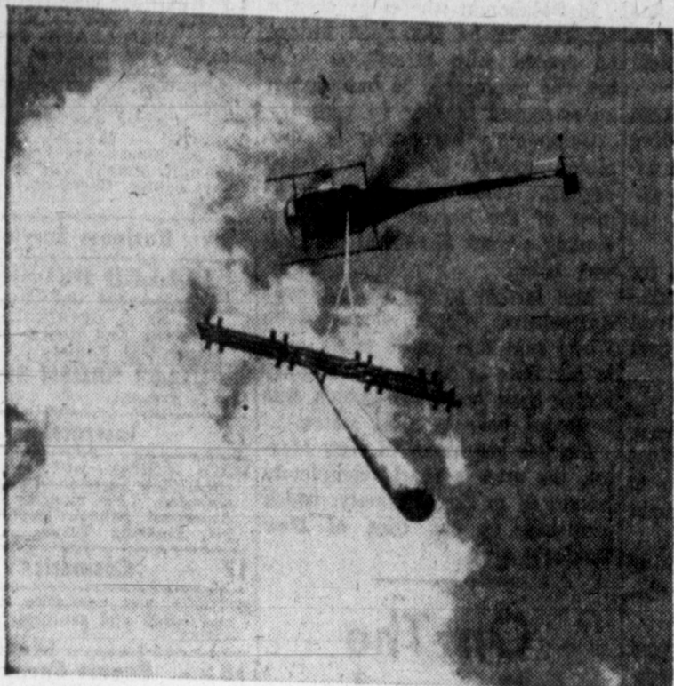
SUSPENSION —It took a helicopter to conquer an almost impassable stretch of northern Idaho mountain terrain when a mile of long distance telephone line had to be relocated. Up and over the cliffs she went, with a phone pole blithely floating along.
