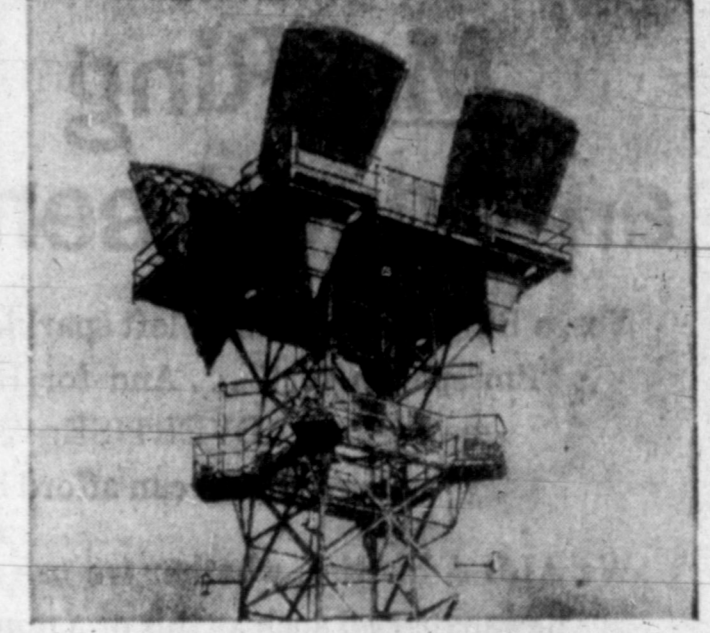
NEW MICROWAVE TOWER supports "cornucopia" antennas that beam Long Distance messages, television programs across Southwest. Capacity of many present microwave antennas is also being expanded to provide additional pathways for growing volumes of Long Distance conversations.
