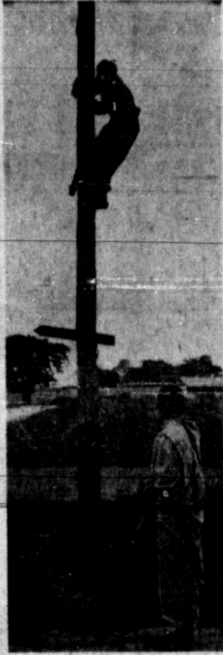
UP HE GOES —Although it is torn by civil war between government forces and pro-Communist guerrillas, war and peace combine to share the scene in Vientiane, capital of Laos. A soldier is climbing a telephone pole to repair damaged communication wires, as Buddhist monk watches.
