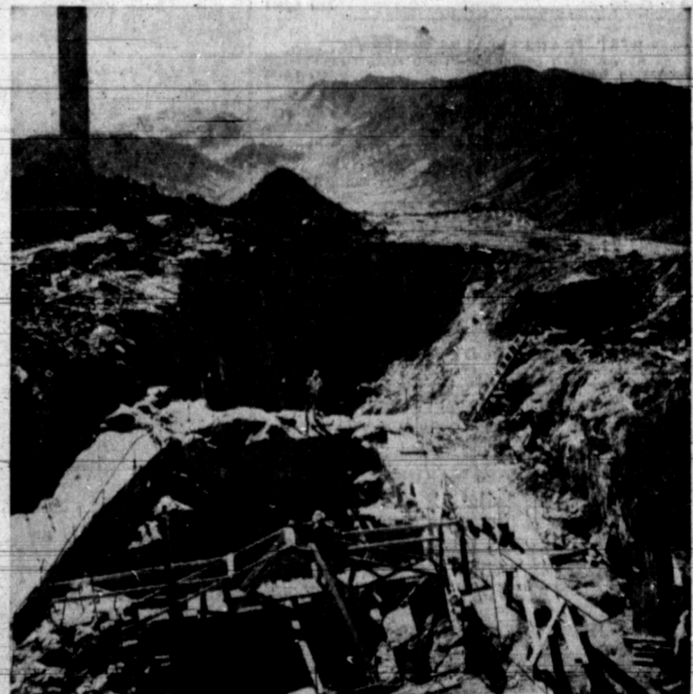
IN REVERSE —Digging a hole in the ground seems an odd way to reach for the sun, but that's what is happening at Kitt Peak National Observatory in the Quinlan Mountains of Arizona. Site of the world's largest solar telescope, the giant hole will contain an observing room where scientists will work to learn more about the sun.
