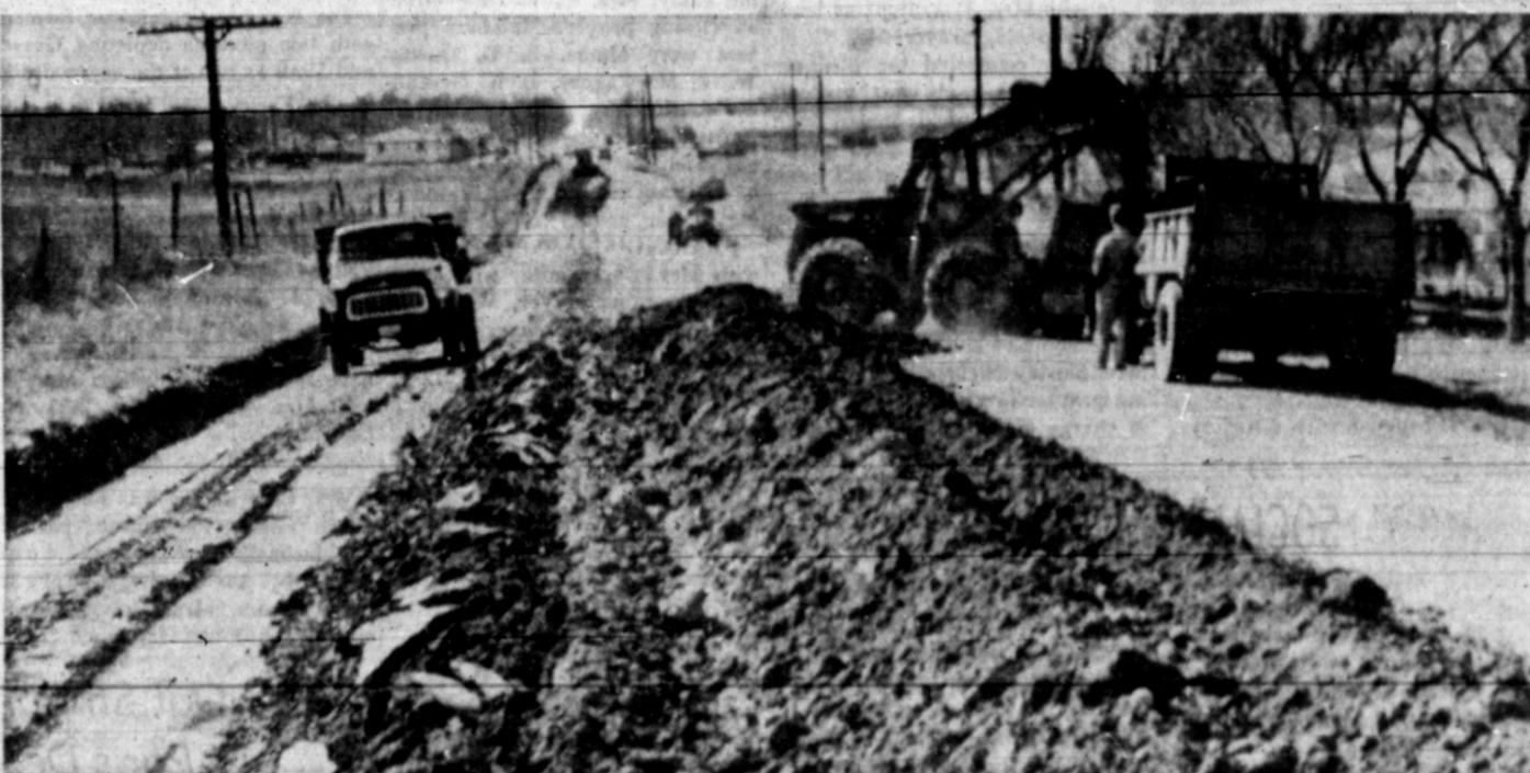
HIGHWAY TO PROGRESS — This is a typical scene of modern advancement that will be found in many places throughout Pampa and Gray County this Spring and Summer as road and street improvements are carried out. The picture above was taken by a Pampa News photographer as work gets under way on a one-half mile stretch of E. Browning St. from Jupiter St. east to the end of Browning. The joint city-county project will result in the widening of the thoroughfare to 37 feet from its present two-lane roadway to better take care of the increasing traffic. (Daily News Photo)
