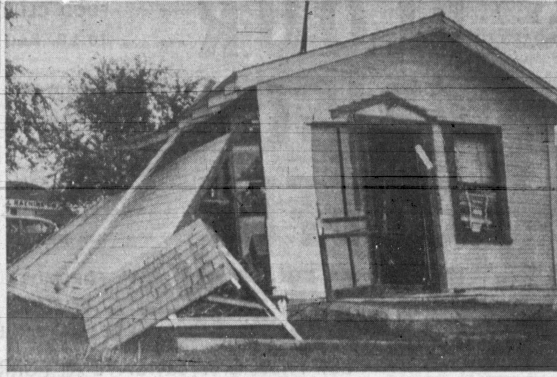
EXPLOSION RESULT — Gas which accumulated under this office building of the H. H. Heiskell Machine Shop, 917 W. Brown, early this morning exploded, sending the owner to the hospital with broken ribs and facial and hand burns, and ripped the building apart. The left wall, shown above, was blasted out as were windows and doors. (Daily News Photo)
