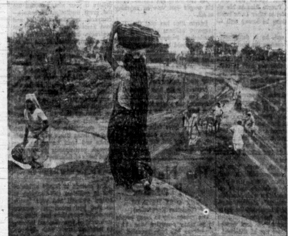
THE ROAD AHEAD —With crude baskets, shovels and bare hands as their only tools, women join their men in building a road to link the main highway with a village near Baroda, in India's Bombay State. The government pays workers for the improvement project, part of a plan to raise living standards in India.
