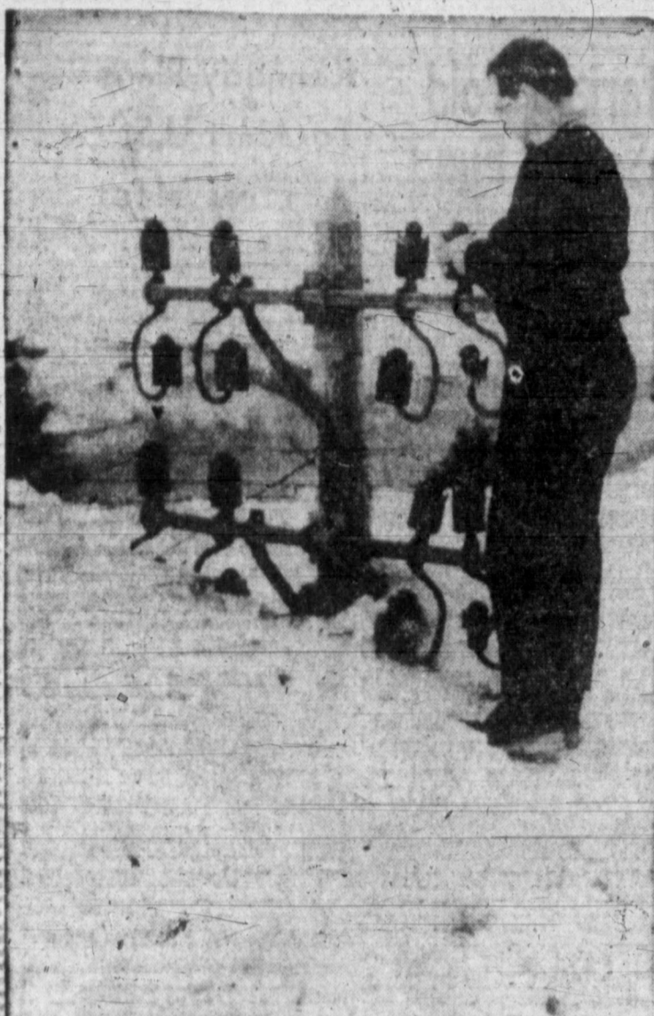
THE SNOW IN FRANCE —The telephone lineman in Chamrousse, France, doesn't grumble about the weather. After a heavy snow and severe drifting, he was able to walk right up to the insulators and make his repairs. Chamrousse is a winter resort in the French Alps.
